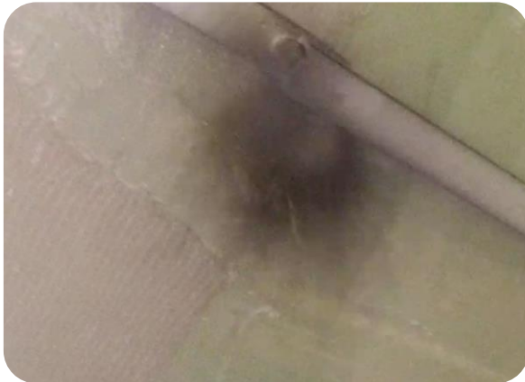
FLASH OVER DAMAGE RELATED TO DAMAGED DOWN CONDUCTOR CABLE
