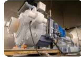
Cold start-up testing gearbox
