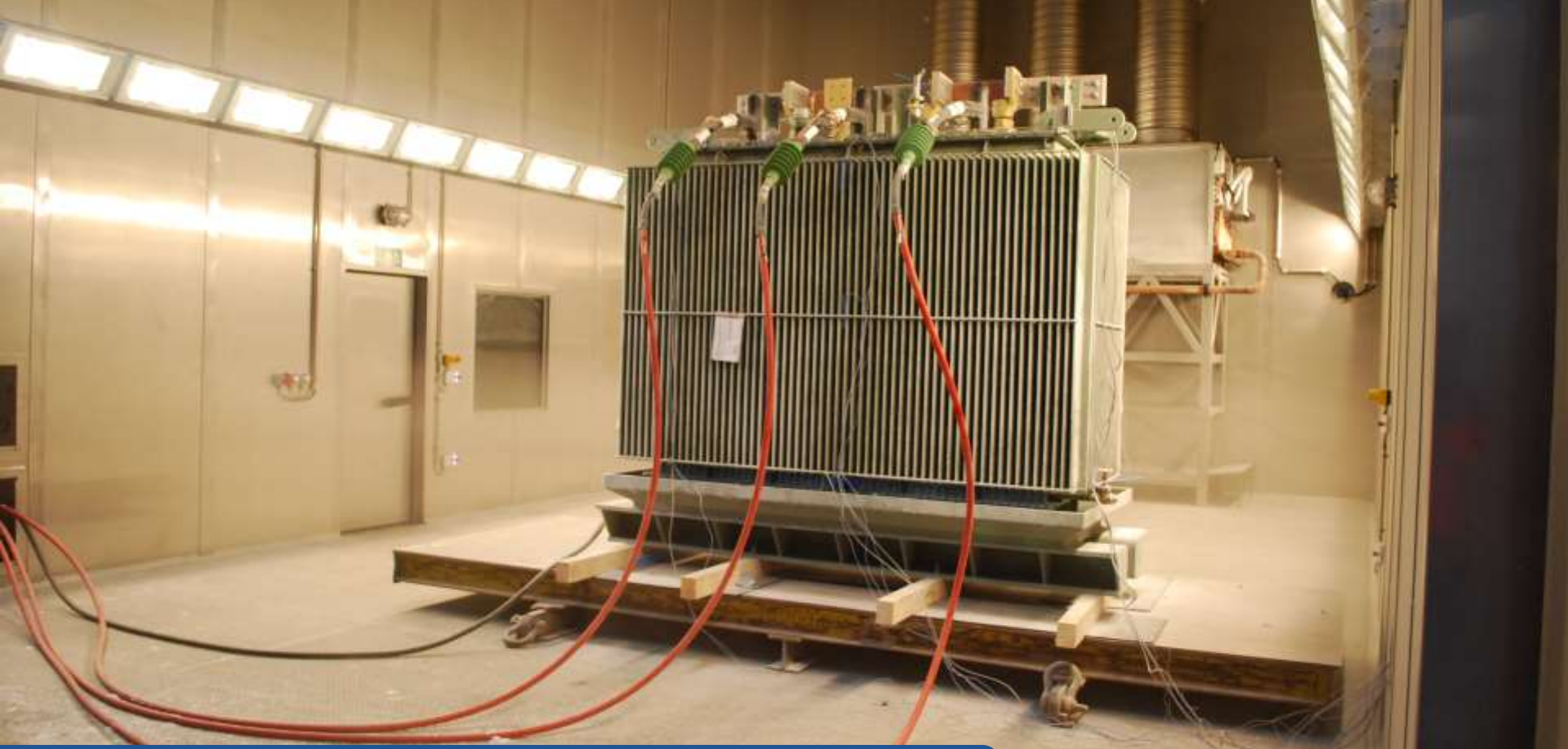
Case story: wind turbine transformers
