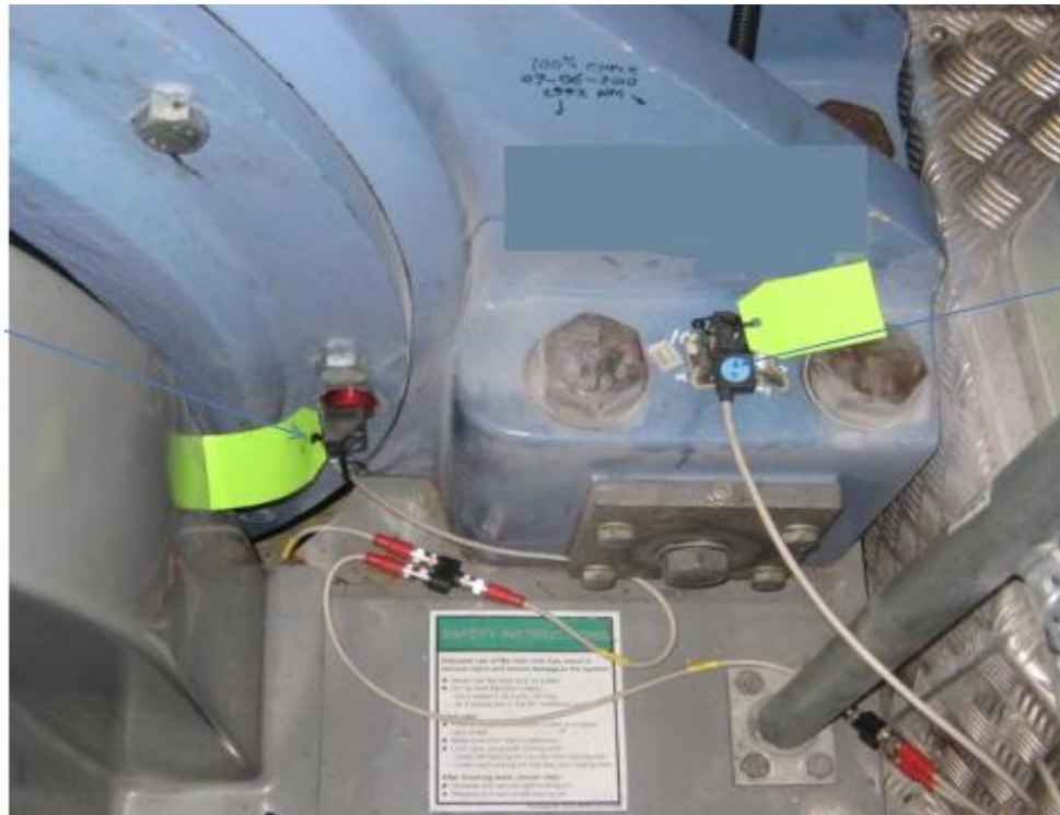
2 axis Nacelle Sway Accel
