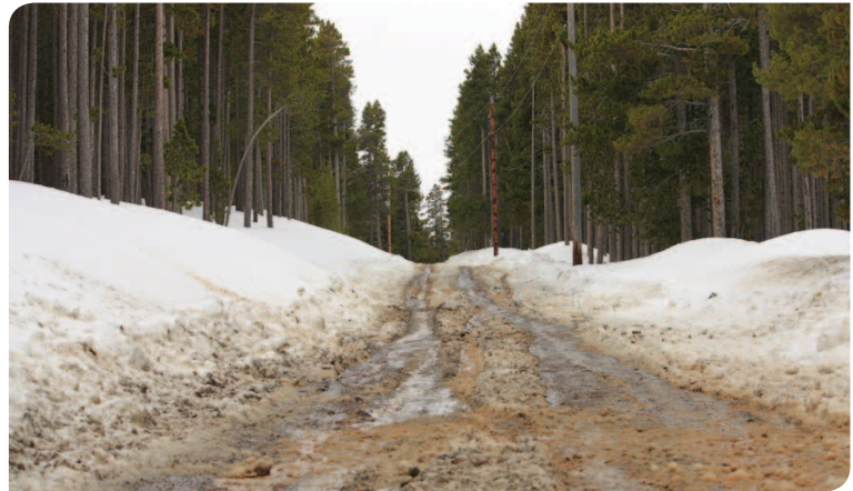
Figure 10. Thaw weakening of a gravel road.
