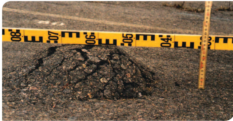
Figure 9. Example of stone lift under pavement caused by frost heave.
