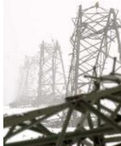
Fig. 3: Damaged power line poles in Münsterland area on 26.11.2005 (Photo © DPA, 2005; see [2] and [3] for more information)
