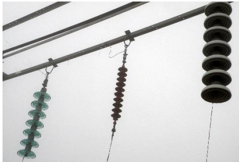
Figure 2. Arrangement of insulators
