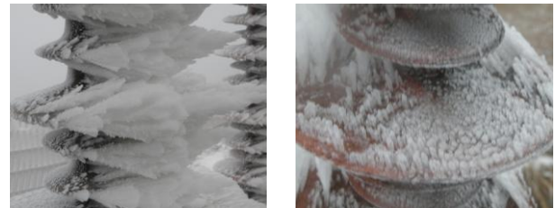
Figure 8 Appearance of ice-covered insulator at XMNTB
