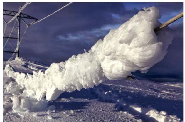
Figure 1: In-cloud icing on a power line (Photo Ole Gustav Berg/Statnett)
