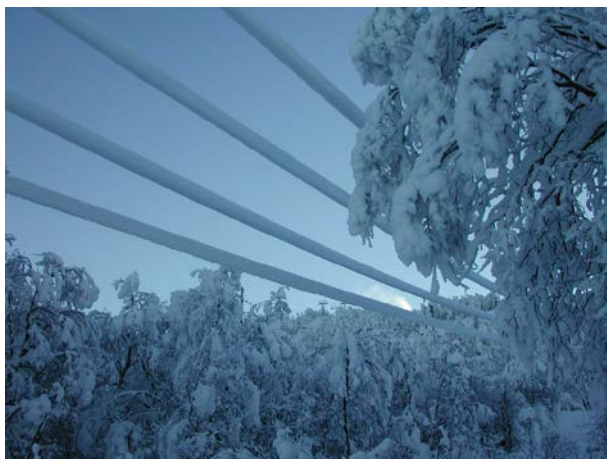
Figure 2: Snow load on power line (Photo Hallingdal Kraftnett)
