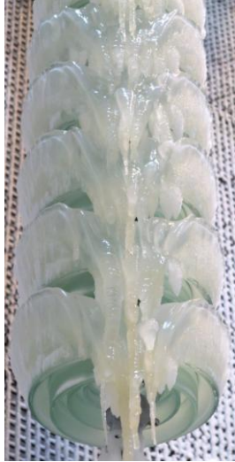
Figure 8: View of the insulator string covered by glazed ice.
