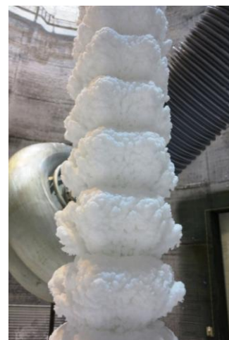
Figure 7: View of the insulator string covered by rime ice.
