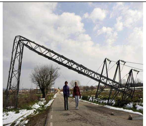
Fig 05 : Tower of 25kV line , 2 circuit, collapsed by the weight of the snow
