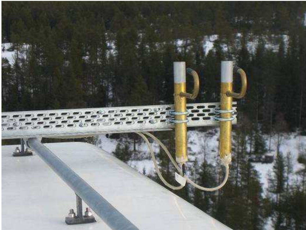
Fig 2 Ice Sensors installed on wind power plant
