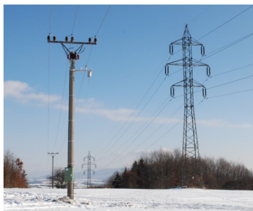
Figure 1: Monitoring station PMS installed on MV line
